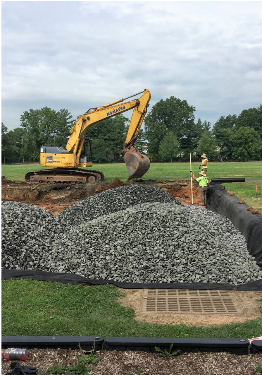
Professional contractor grading the topography of a restored wetland (Photo Credit: Brooke Maslo)
