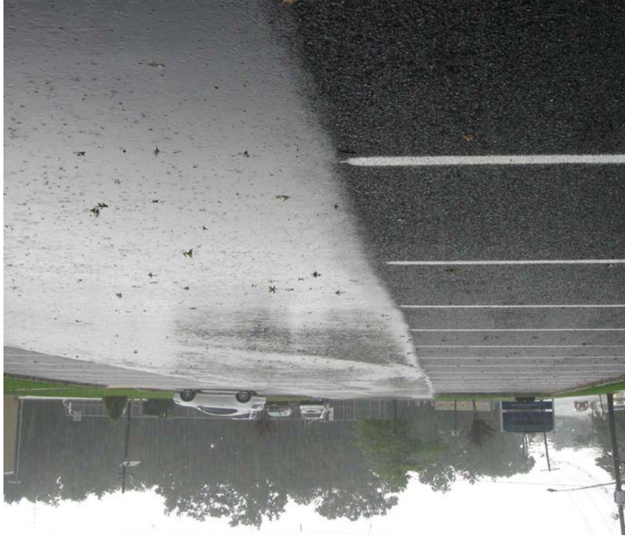
Porous asphalt parking spaces adjacent to conventional asphalt driving lane (Photo Credit: Rutgers Cooperative Extension)
