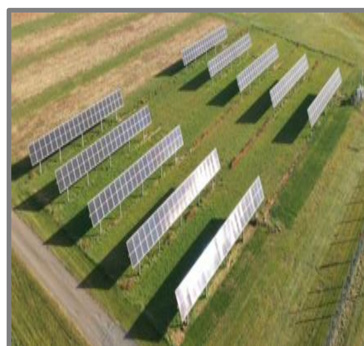
A single-axis tracking array at ground level. Image from Advanced Solar Products.
