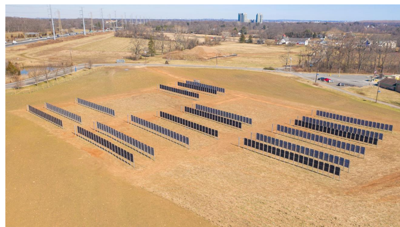
Overview of the site right after the installation of the solar panels
